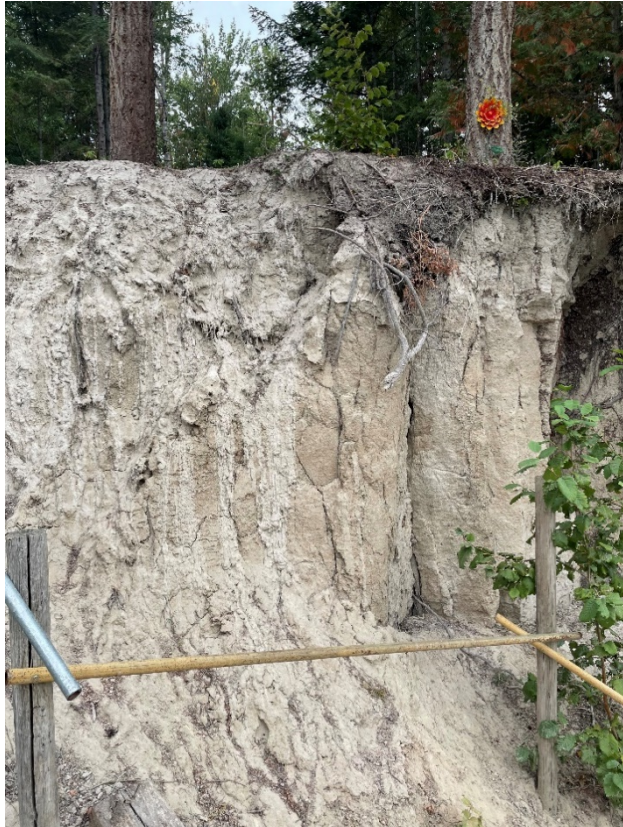
Ricco Property: Clear evidence of steep slopes and mass failure
